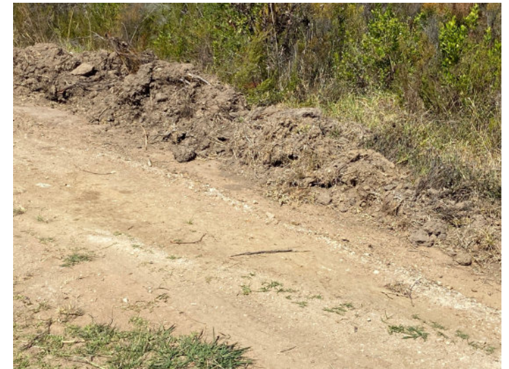
//11 Zero progress on rehabilitation of road edge as promised (below)
