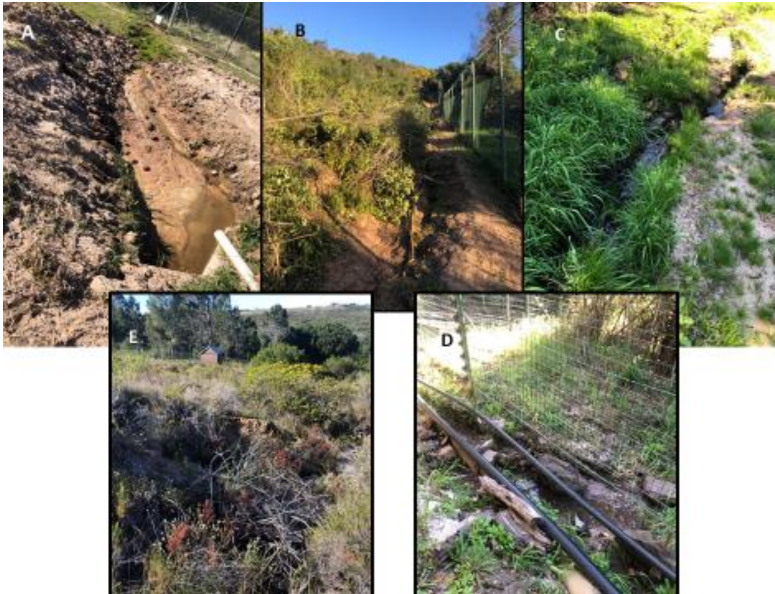
Photograph panel 3. Illustrates A. Recently opened storm water culvert; B. Erosion runnel on steep slope along northern fence line; C. Erosion runnel down a path in southeast section of Estate; D. Erosion down a path along southeast fence line; E. Erosion donga formed at storm water outlet near southeast corner of Estate.
