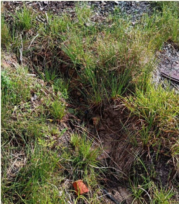
Erosion due to storm water outlets in block 6.
